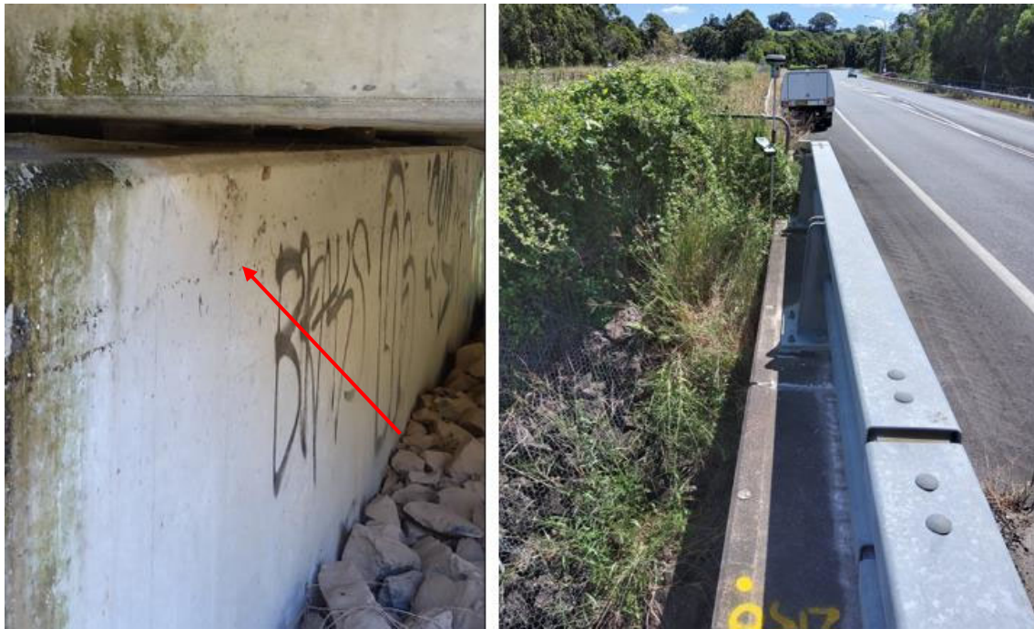
Figure 19: Debris on underside of bridge structures, requiring vertical offsets.
