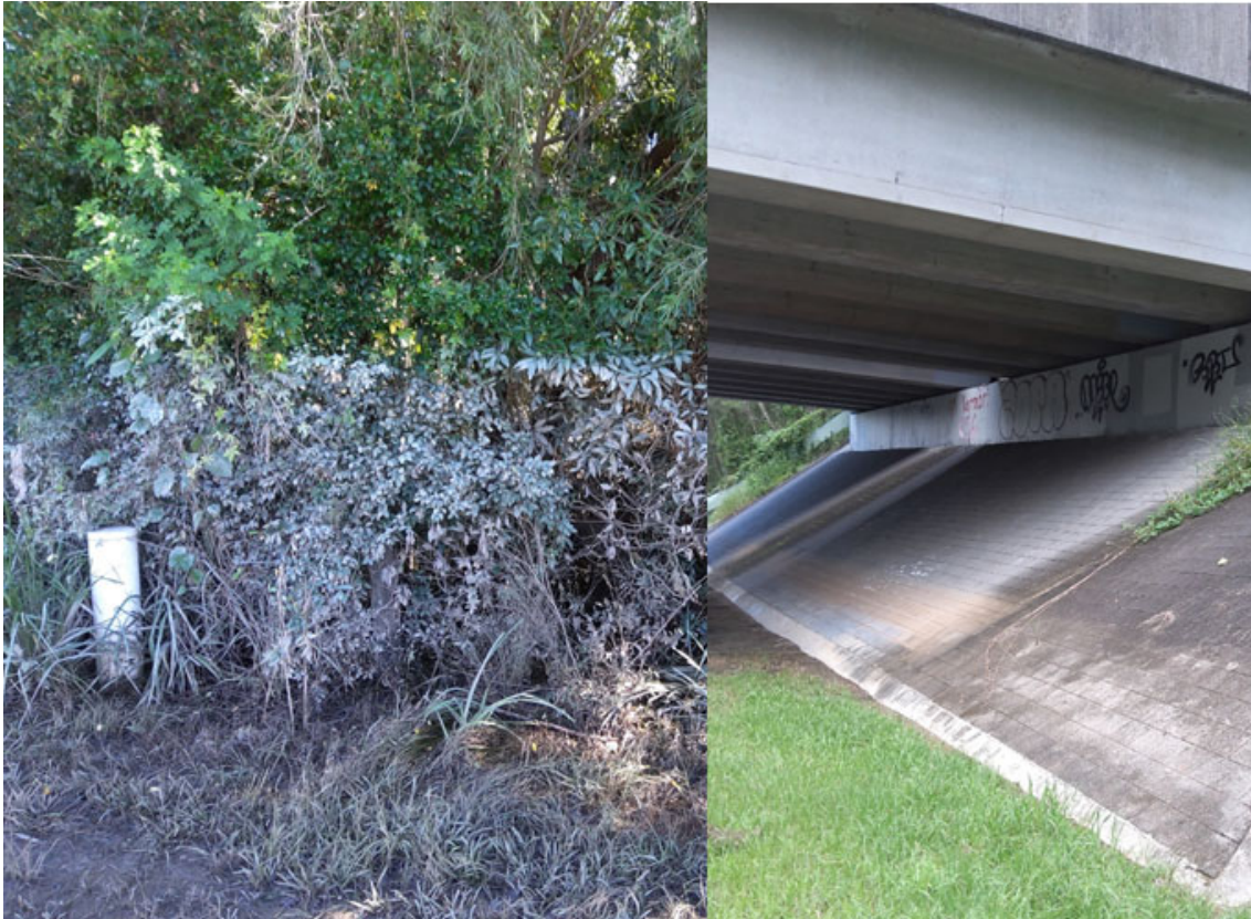
Figure 14: Silt line on vegetation and structures.
