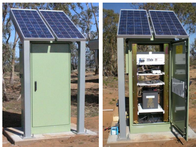
Figure 1: Enclosure with solar panel doubling as a shade awning at a CORSnet-NSW site (Tier 2).
