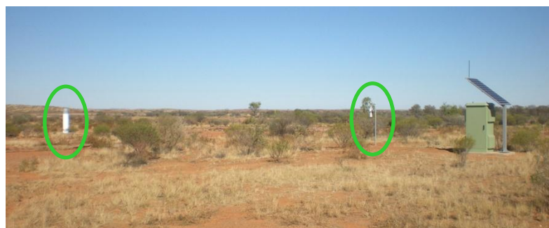
Figure 14: GNSS CORS pillar, automatic weather station and solar power with backup battery power installation at a CORSnet-NSW site (Tier 2).
