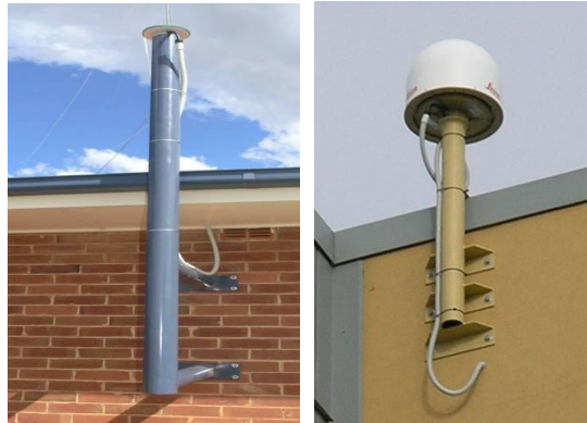
Figure 5: Powder-coated antenna monuments at CORSnet-NSW sites (Tier 3), also showing the use of steel ties, waterproof connectors and partial drip loops.
