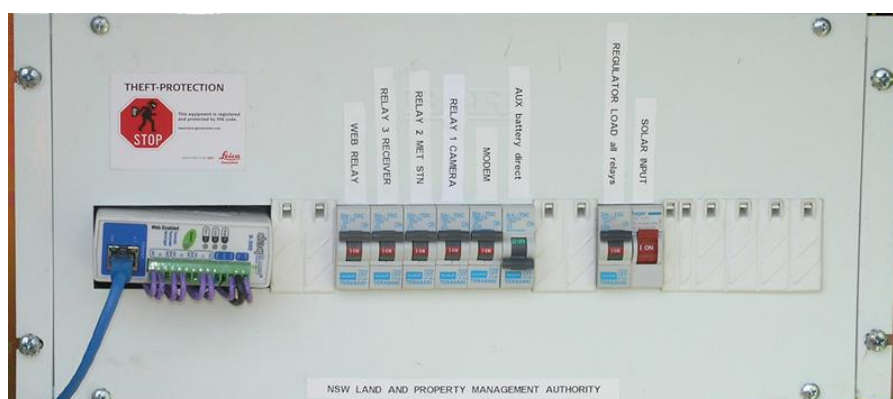
Figure 15: Labelled circuit breakers at a CORSnet-NSW site (Tier 2).
