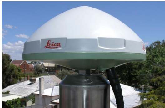
Figure 7: Antenna monument with bevelled edge at a CORSnet-NSW site (Tier 3).
